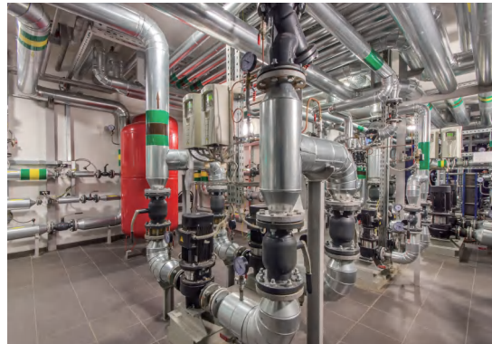
Municipal heating system
